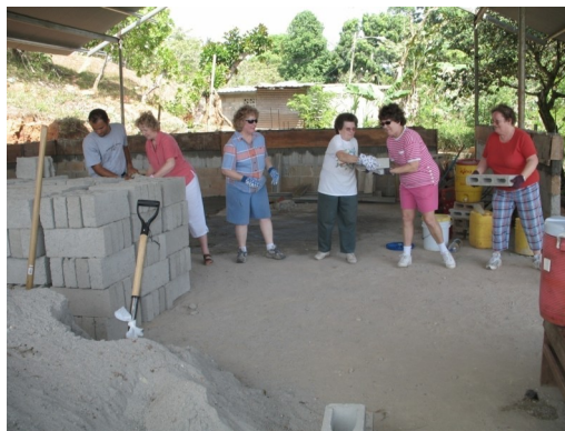
Jane Lute, center, wearing blue shorts, was part of the block line getting materials into the new church building. Moving building materials from the street to the construction site is a major effort in less developed countries. The cement blocks were brought up from the street by passing them hand to hand up the hill to the new building.
