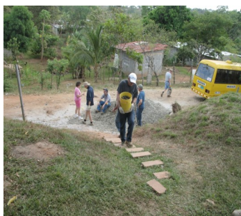
Rob Lute carries a bucket of gravel from a pile in the street of rural Paso Blanco, Panama. All the sand and gravel had to be hand-carried to the construction project for hand-mixing into mortar or concrete.
