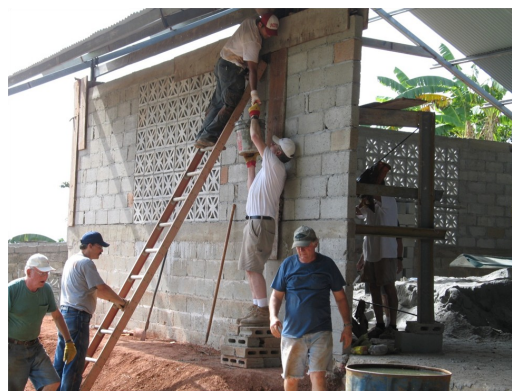
The Work and Witness team worked together on the new church building, using their individual skills and talents to improve the community by providing a place of worship.
