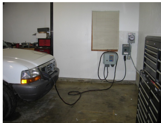
The truck is plugged in and charging.
