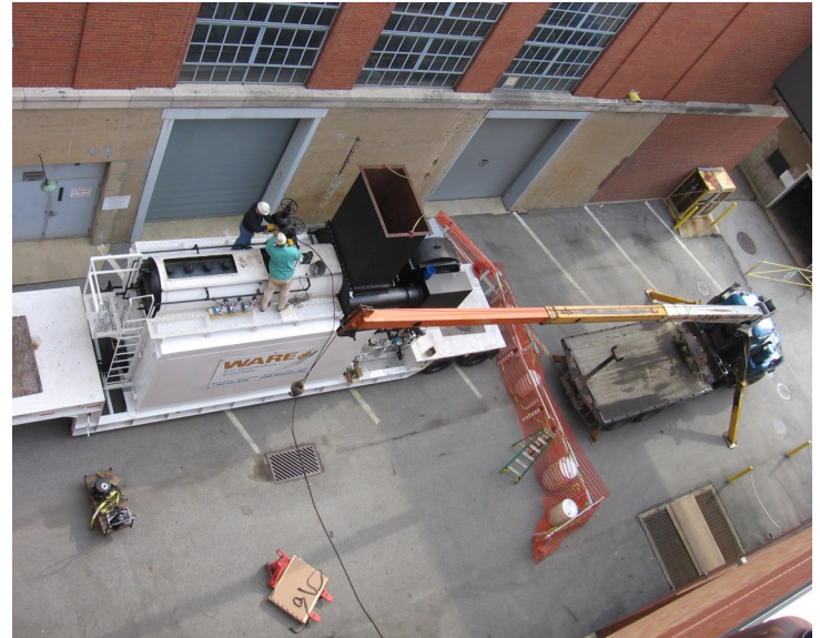
Co-gen employees Steve Rebovich and Brent Culp work on getting a temporary boiler set up near the S. W. Jack Cogeneration Plant. This unit will provide an alternative source of steam for the campus while repairs are made to the 150 foot brick stack at the power plant.
