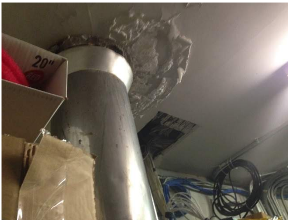
Ceiling Damage, Mechanical/Electrical Room
