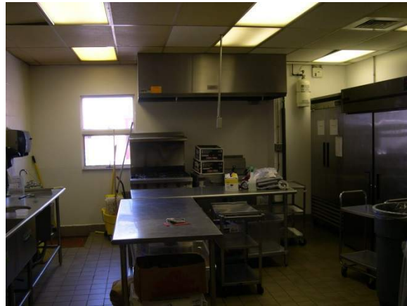
Prep Areas, Issuing Kitchen
