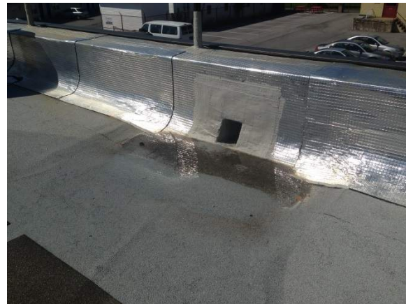
Water Pooling near Existing Roof Scupper
