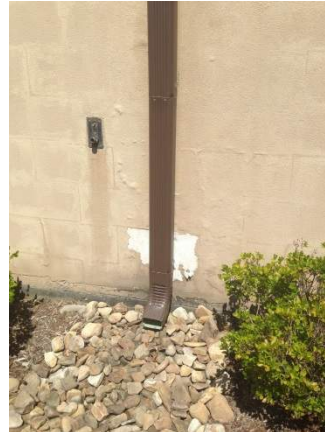
Damaged Stucco at Downspout
