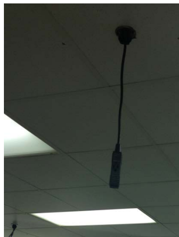
Detail of Power Strip Hung from Kitchen Ceiling
